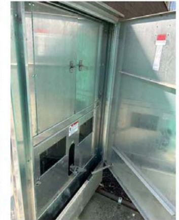
08 Generator Main Switch Enclosure
