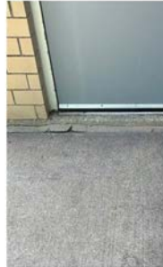
Photo 2: View of exterior concrete settling
