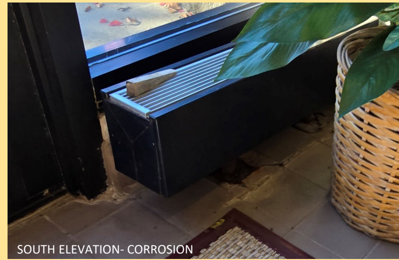
SOUTH ELEVATION- CORROSION
