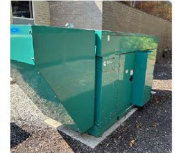
07 Onan Backup Emergency Generator
