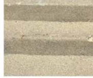
Photo 4: View of exposed rebar at spalled concrete due to corrosion
