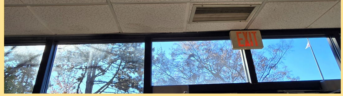
SOUTH ELEVATION- WATER INFILTRATION
