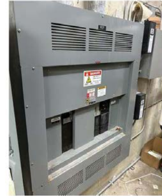
05 Main Distribution Panel MDP
