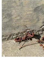
Photo 3: View of spalled concrete due to damage
