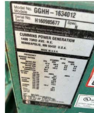
06 Outdoor Generator Nameplate
