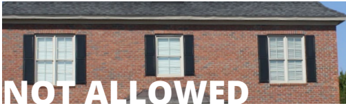
Inappropriately Scaled Shutters.
